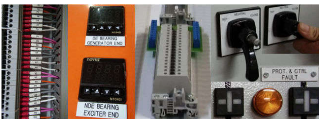
Fig. F Temperature Controllers for Winder Motors Armcoil Armature Re-winder / Mines. Emergency Switches, LEDs, Tile Semaphores
