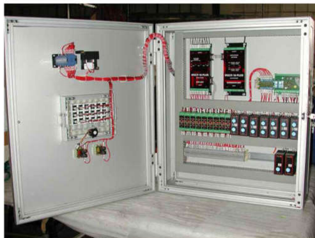
ZAMBIA COPPER MINE Multi-16 with timer modules all in wall mounting Alutech box.
