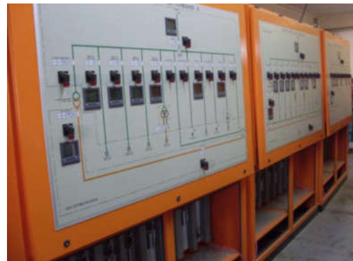
BELOW: South African Control Board in a Stainless Steel Orange Powder Coated Panel.
