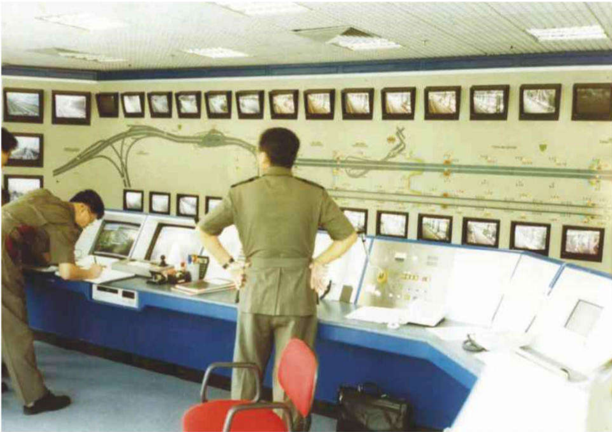
Control Desks with Console and Mosaic Mimic Panel of Route to Hong Kong Airport 1996-1997
