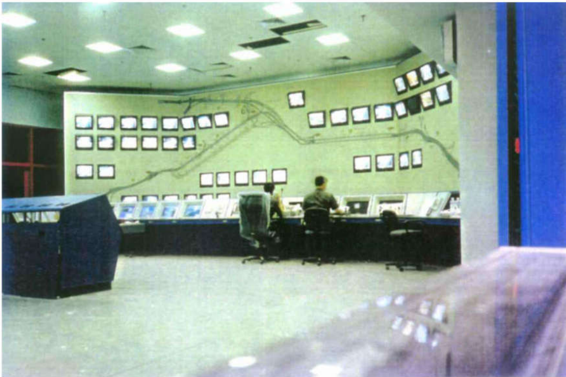
Control Desks with Console and Mosaic Mimic Panel of Route to Hong Kong Airport 1996-1997
