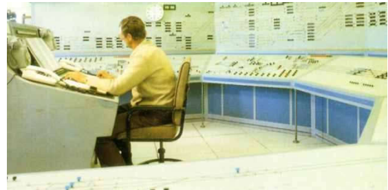
Fig. B shows the practicality of our tailor made console desks (rail control)
