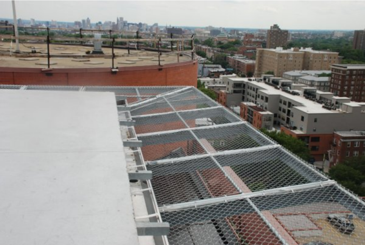
Roof-top Helipad Safety Net
