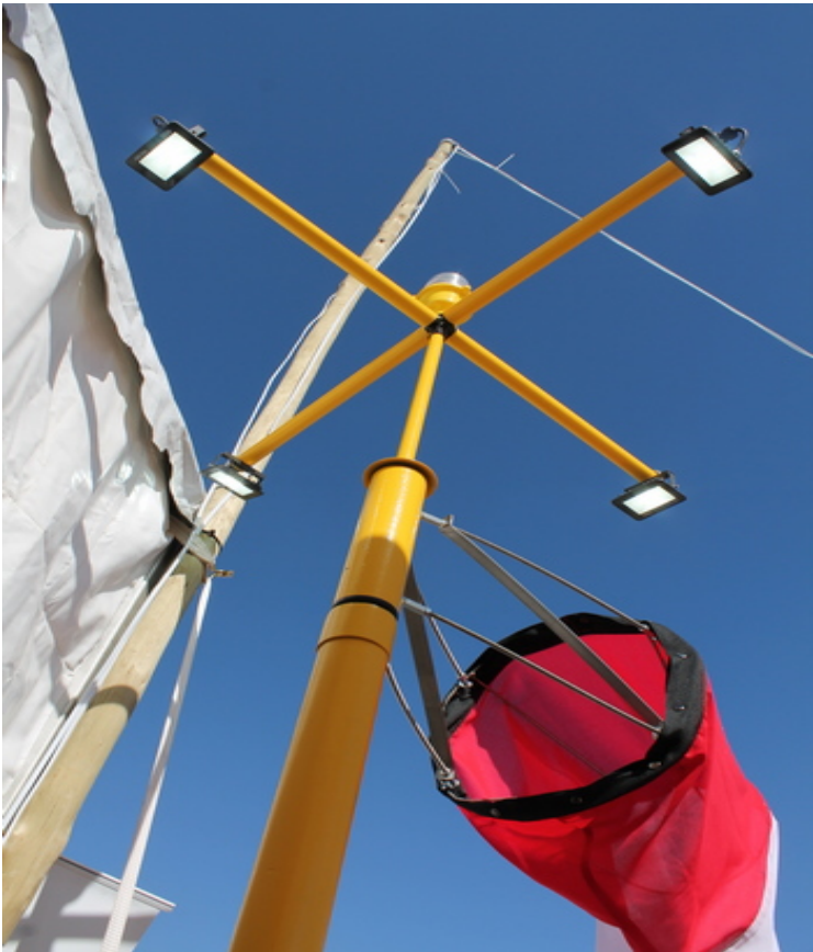
Red & White Strip Windsock attached to pole with flood lights.
