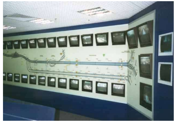
Fig. A shows the convenience of fitting monitors directly into our mosaic (Hong Kong airport bridge)
